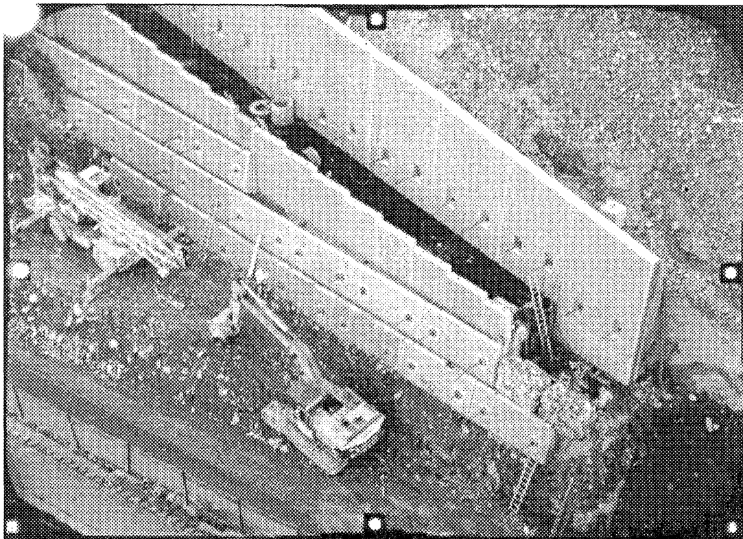
Figure 6 300mm UMK photograph taken from high level close in position - epoch 1 (Note obstructions owing to construction plant)
