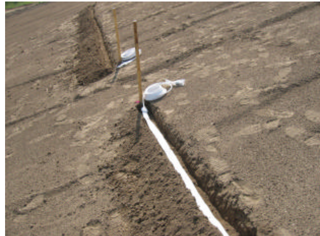
Figure 6: Installation of TDR Sensor cables on a dump-site to monitor the sealing layer.
