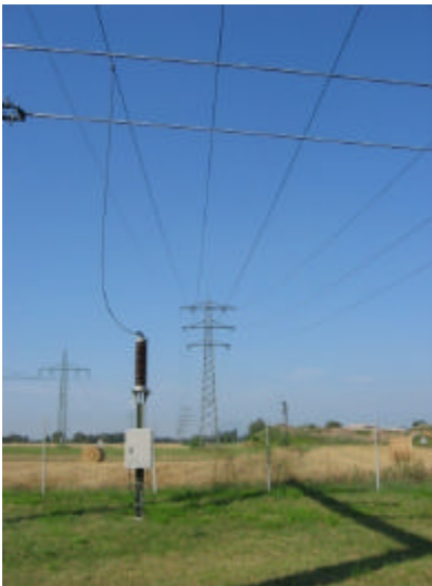
Figure 9: Signal coupling of the low voltage signal to the high voltage power line using a capacity post of the TFH-equipment
